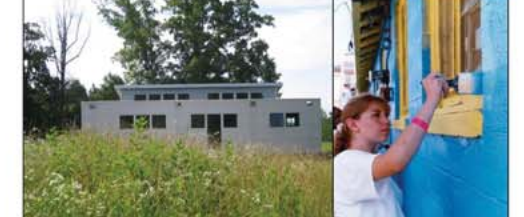
L. ENHANCE EXISTING COOK SHACK The existing cook shack is in poor condition, and as a result is rarely used. There is an opportunity to engage the community in the clean up of this facility.
